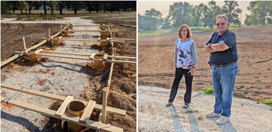
Betty Bittner and Board member Don Schweiger review the Ivy Tunnel foundation layout.
